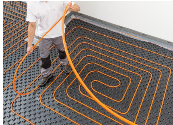
Hot water under-floor heating
